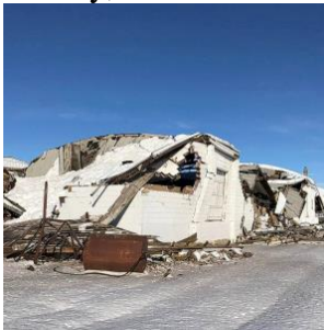
Local buildings collapsed around town
